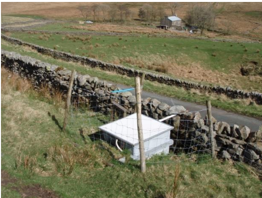
Storage tank with old posts Photo Credit: Ray Duffy
